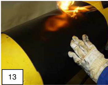
13 Stick the sleeve all the way around the pipe overlapping onto the underlap. Warm up the overlapping area.
