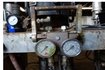
(Part A and B pressure gauges)
