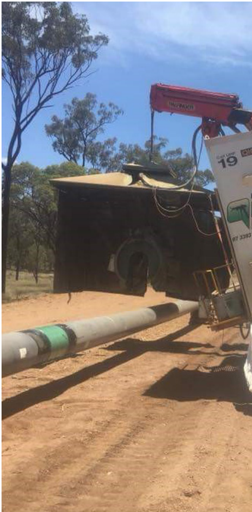
QIC's Automatic Field Joint Coating unit on the move to complete the next FJC.
