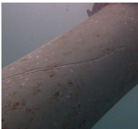
Damaged subsea tripod leg coating requiring protection.
